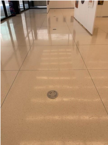
One of the two rows of floor outlets.
