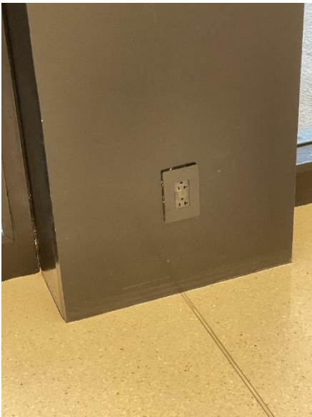
One of the 4 wall outlets located on the north side of the pillars.
